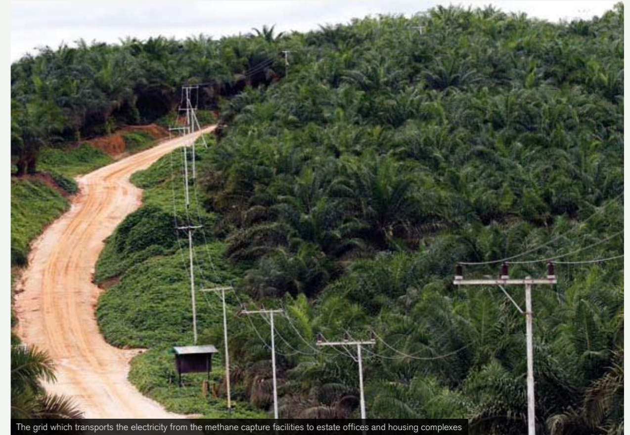
The grid which transports the electricity from the methane capture facilities to estate offices and housing complexes
