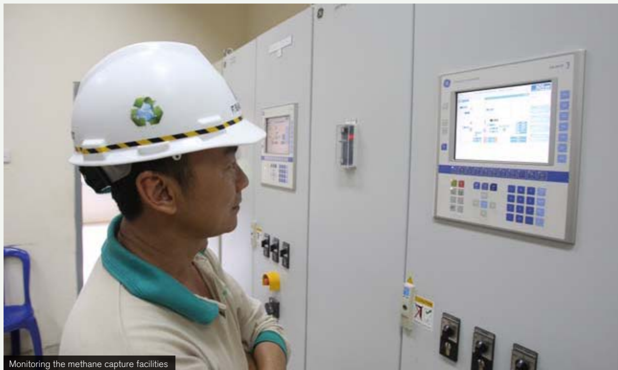
Monitoring the methane capture facilities
