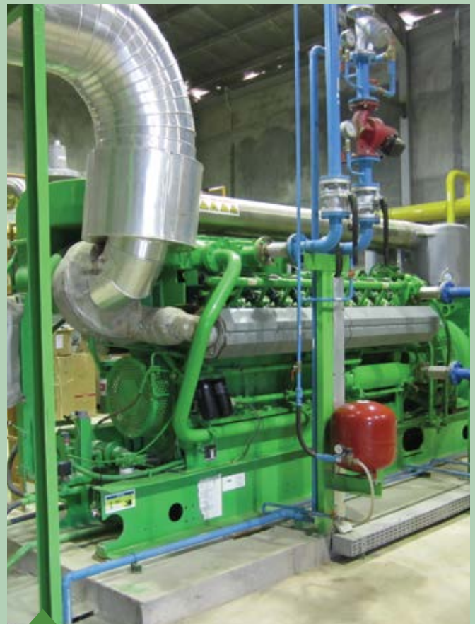
One of the biogas engines used to convert methane to electricity
